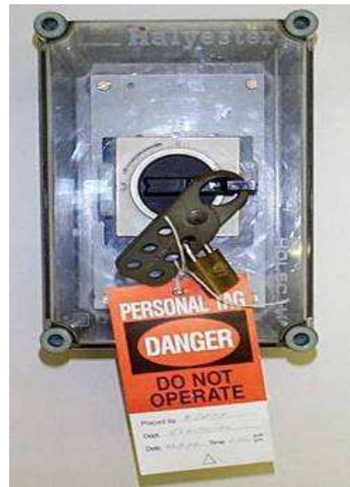
Figure 7. Danger Do Not Operate Tag and Lock
