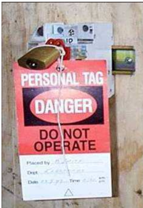
Figure 6. Danger Do Not Operate Tag and Lock
