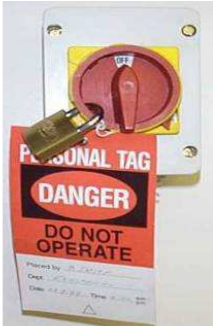
Figure 8. Danger Do Not Operate Tag and Lock
