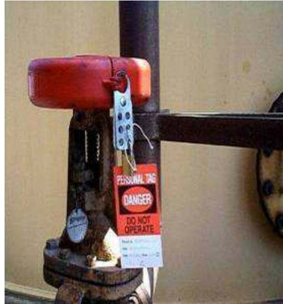
Figure 9. Safe Isolation for Steam Valve Using Callipers
